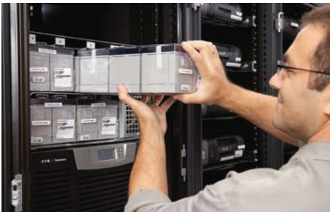
IT staff can easily replace battery modules.
